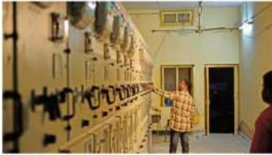
Through the app the consumers will be able to report power outages and its location Photo: Pradeep Gaur/Mint
